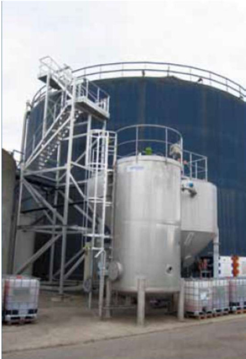
P-recovery (struvite) from digested sludge – Leuven, BE
